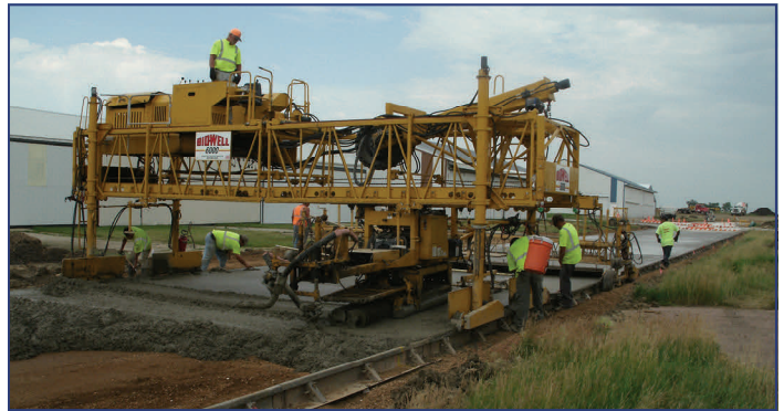
7/12/2011 - D&G Concrete Construction crews laid concrete for the new hangar taxiways at the Madison Municipal Airport. The project finished at the beginning of July. The taxiways are part of recent improvements at the airport.
